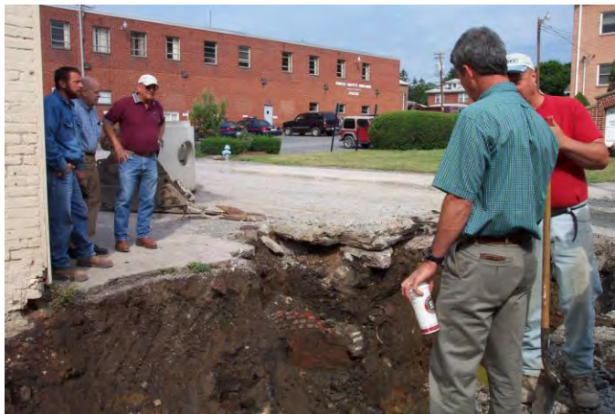
A typical progress review by Public Works Director Chris Hovatter overseeing Frostburg's combined sewer separation program. The work in progress is on Alley 44 at Broadway.
